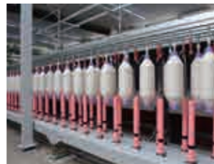
After lifter goes down and grips the full bobbins, loop rail slides half a pitch and the empty bobbins are inserted
